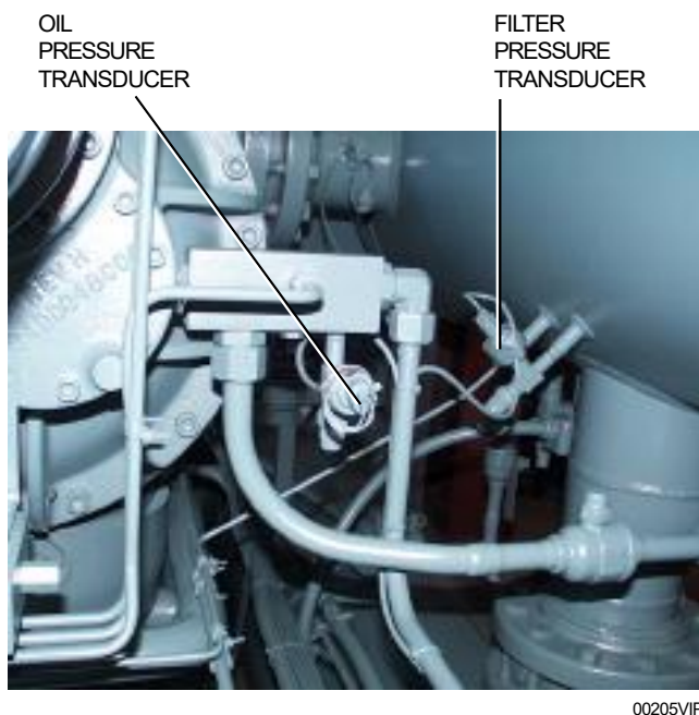
FIG. 18 – OIL AND FILTER PRESSURE TRANSDUCERS
